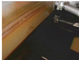
Typical operating gas turbine reservoir
